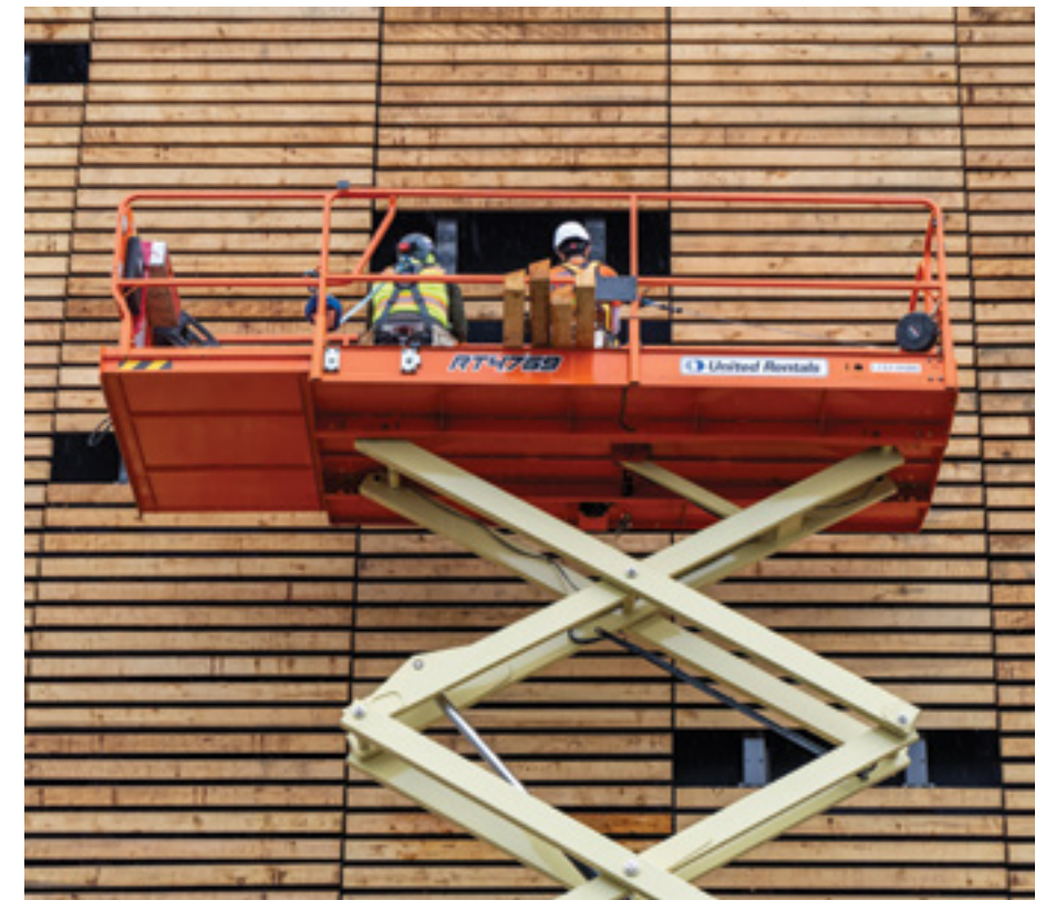
Workers install Alaskan yellow cedar on the west face of the Ocean Pavilion (read more on page 6).
